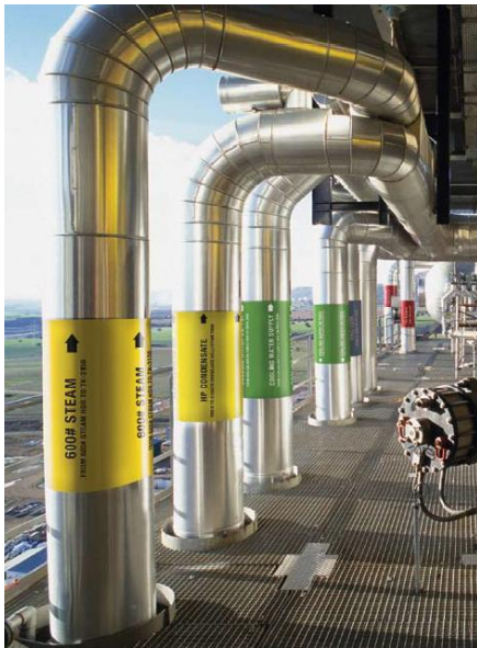
HEAT TRACING / PIPE MARKING
